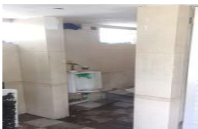
Toilets are damaged
